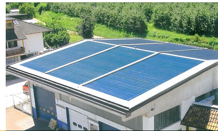
Commercial roof refurbishment with asbestos remediation, thermal insulation and double layer Phoenix SOLAR waterproofing system with twenty-years warranty, 19 kWp General SOLAR PV® building integrated photovoltaic system.
