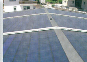
ROOF REMAKE (WATERPROOFING, THERMAL INSULATION AND ASBESTOS REMEDIATION) WITH GENERAL SOLAR PV® SYSTEM
